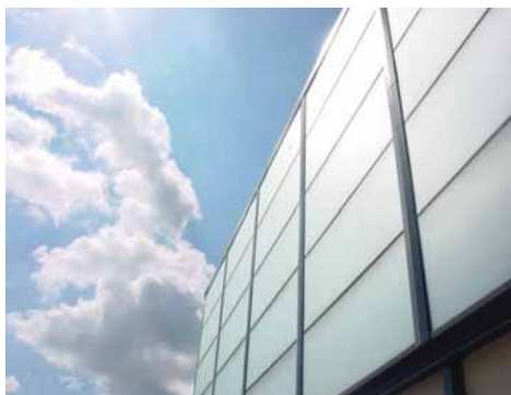
Malmö is also aiming at becoming a SolarCity. This solar panel installation heats the local swimming and sport arena Kockum Fritid in Malmö. Photo: Tor Fossum, City of Malmö
