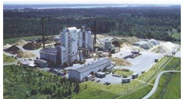
Gasification plant for bio-DME
